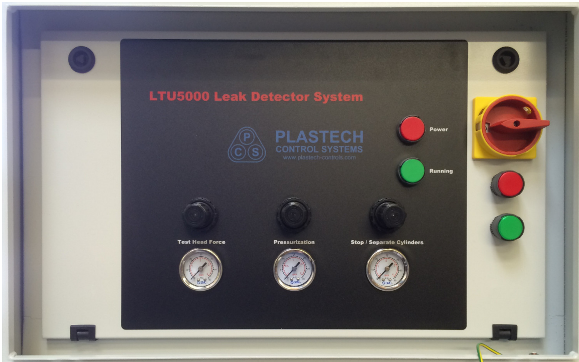
LTU9000 Main Cabinet
